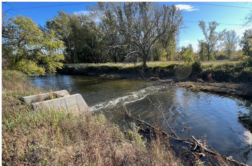
Figure 6-8. Return Flow Outfall Structure at the Root River
