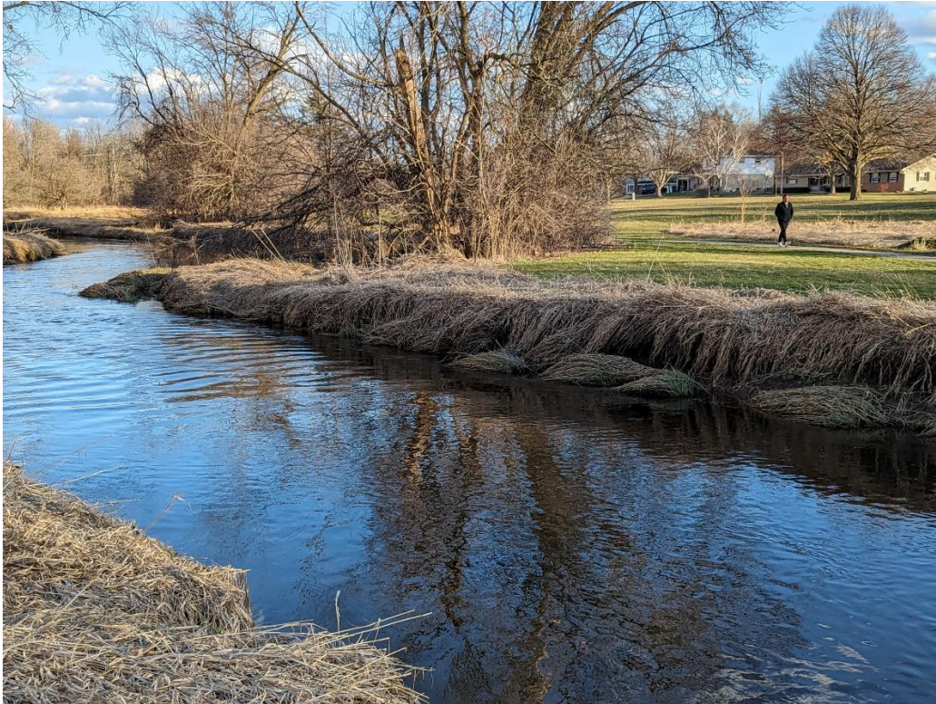
Image 1.3 – Bank on right, undercut, partly covered with grass.
