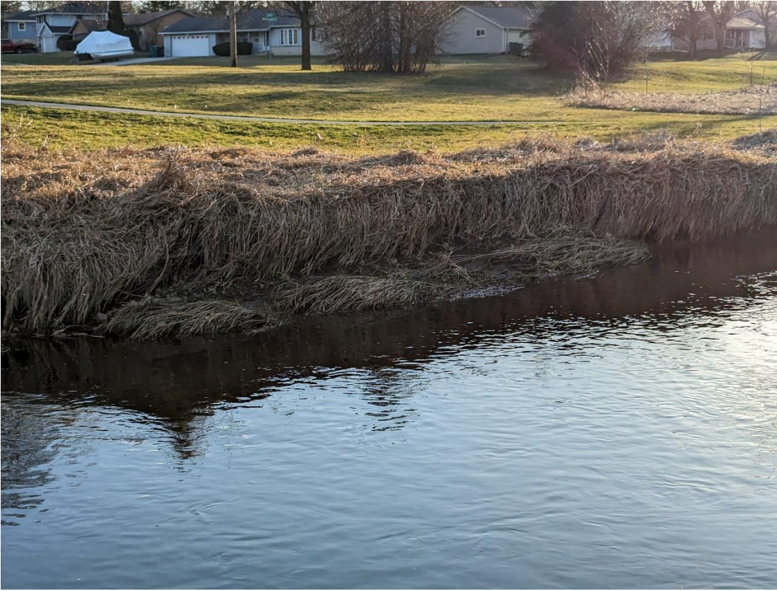
Image 2.3 – Bank, undercut, with slumped sections of soil in water.
