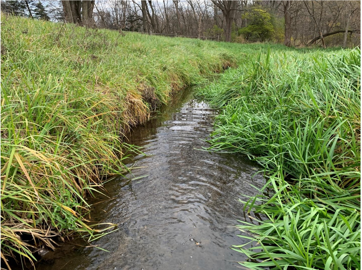
Image 3.1 – Bank, undercut with slump, covered with grass.
