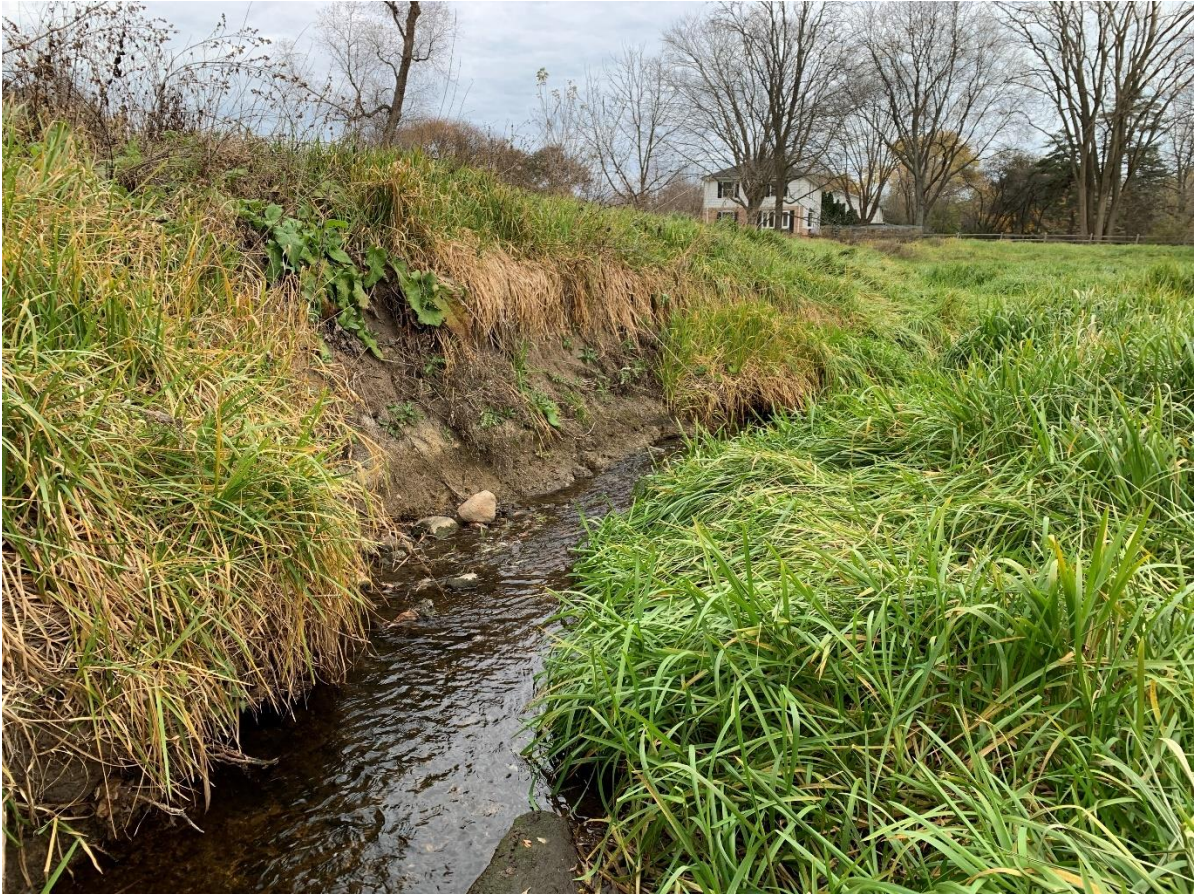
Image 2.1 – Bank, undercut with exposed roots and overgrown with grass.
