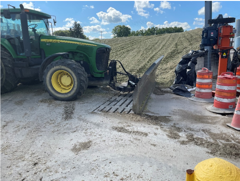
Photo 20: Feed leachate inlet grate in FSA 1 facing south and down.
