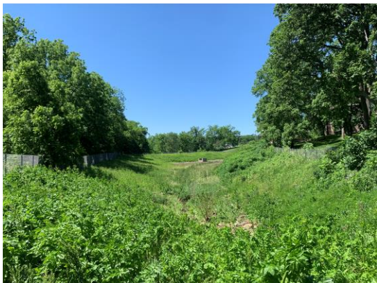
Figure 2.04-5 Mickelson Dry Detention Basin
