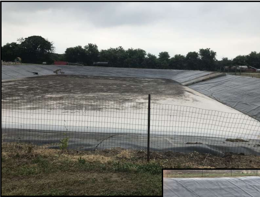
Photo 1 (left): Looking north across WSF 1. A safety fence was observed around the entire perimeter of the storage.
