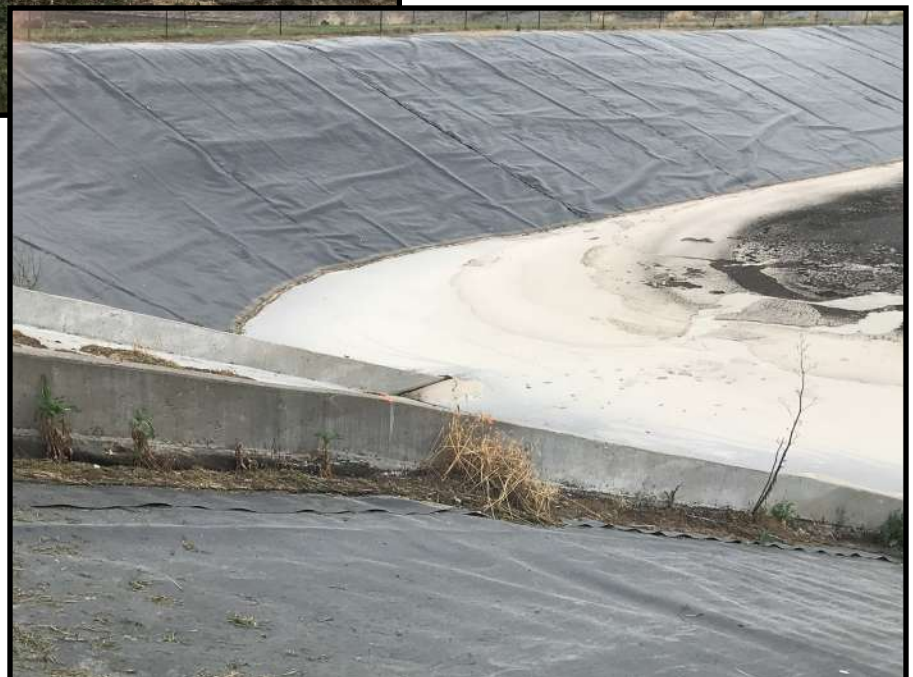
Photo 2 (right): Looking at the concrete ramp in WSF 1. Permanent markers can be seen painted on the concrete in orange.
