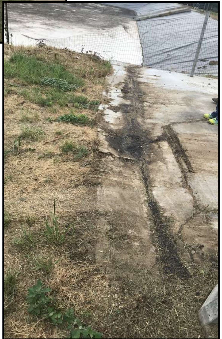
Photo 7 (right): Looking north along the western edge of the solid manure stacking pad pictured in photo 6. A concrete swale was installed along this edge of the pad to direct manure runoff into WSF 1. A clear path of black material from manure runoff can be seen within the swale leading into WSF 1.
