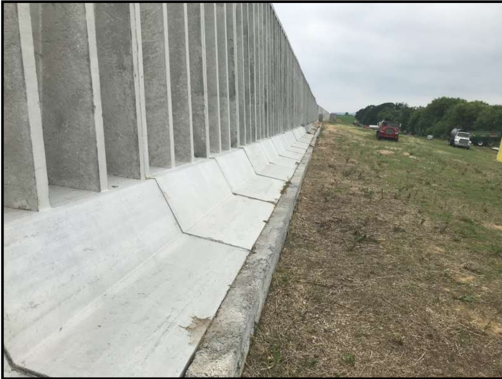
Photo 13 (left): Looking along the northern end of the feed storage area. The wall has been extended along the entire north end to address past issues with leachate flowing off the end of the feed storage area. No evidence of leachate discharging from the north end of the feed storage was observed.
