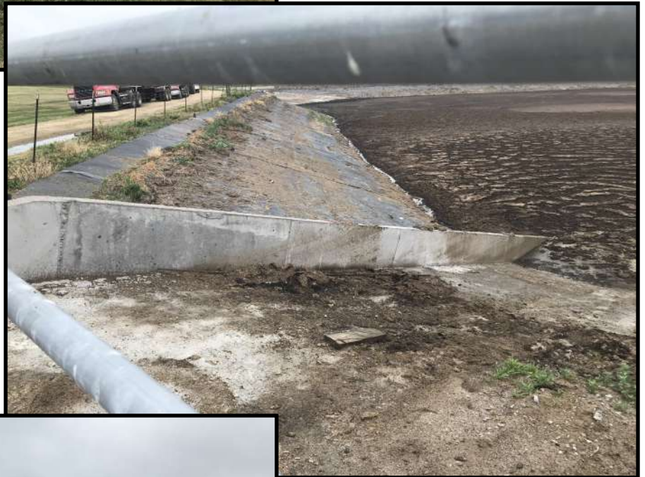
Photo 4 (right): Looking at the concrete ramp in WSF 2. Permanent markers can be seen painted on the concrete in orange.
