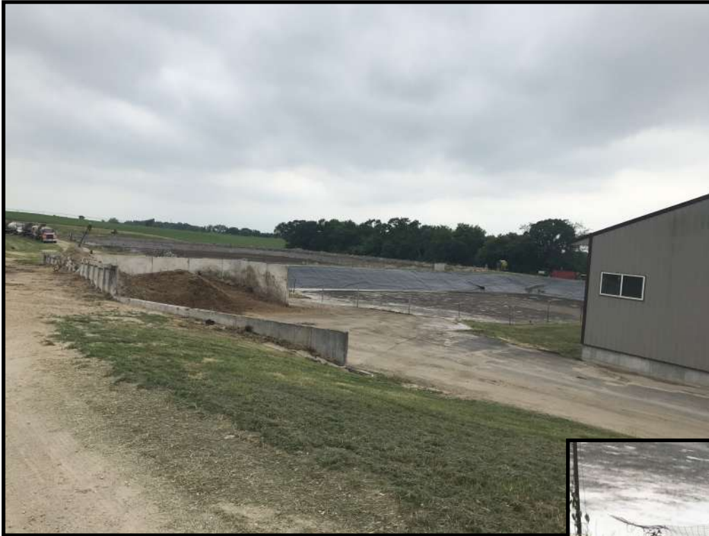
Photo 6 (left): Looking north west at solid manure stacking pad located off of WSF 1. The concrete area around the pad has been expanded to direct manure runoff directly into WSF 1.
