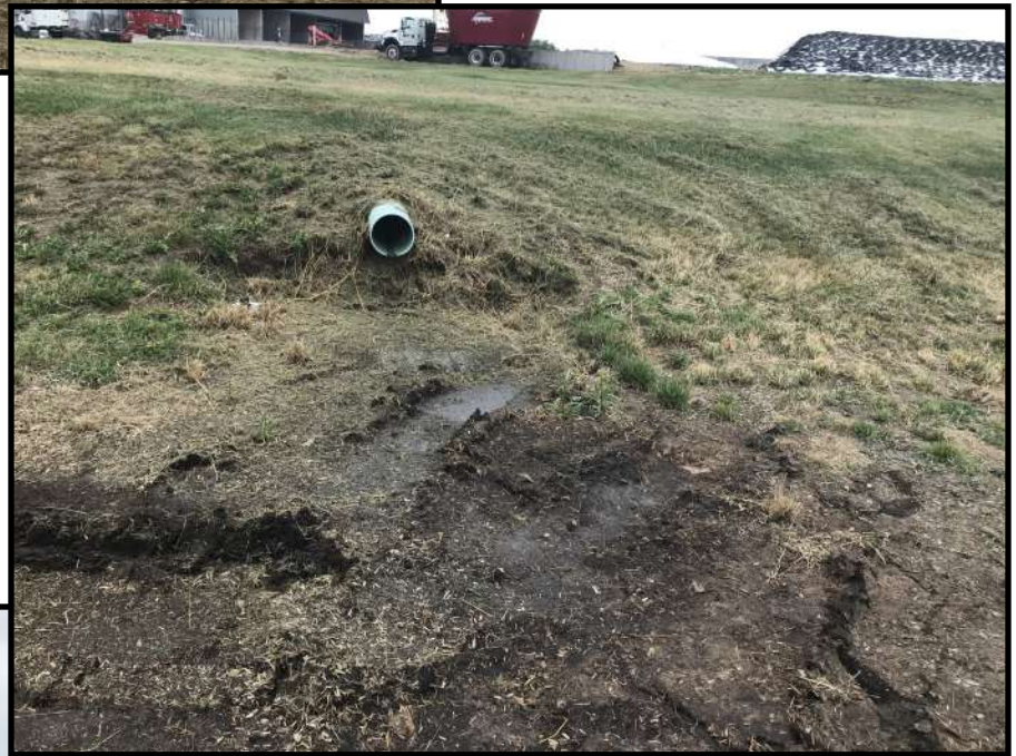
Photo 11 (right): Looking at one of the outlets where feed storage runoff discharges out onto the VTA. Dried debris from feed storage runoff was observed at the base of some of the outlet pipes and was seen accumulating in the area between the outlets and the start of the VTA.
