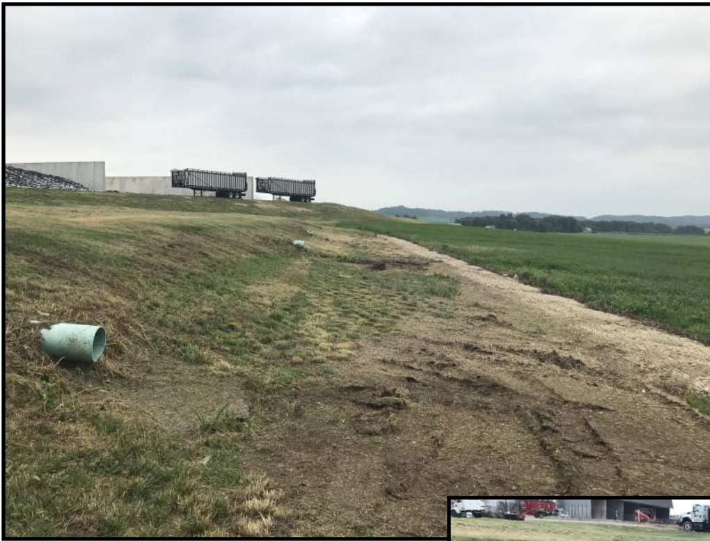
Photo 10 (top left): Looking east along the outlets across the beginning of the VTA. Concrete has been poured at the base of each outlet pipe to prevent erosion and pooling of feed storage runoff.
