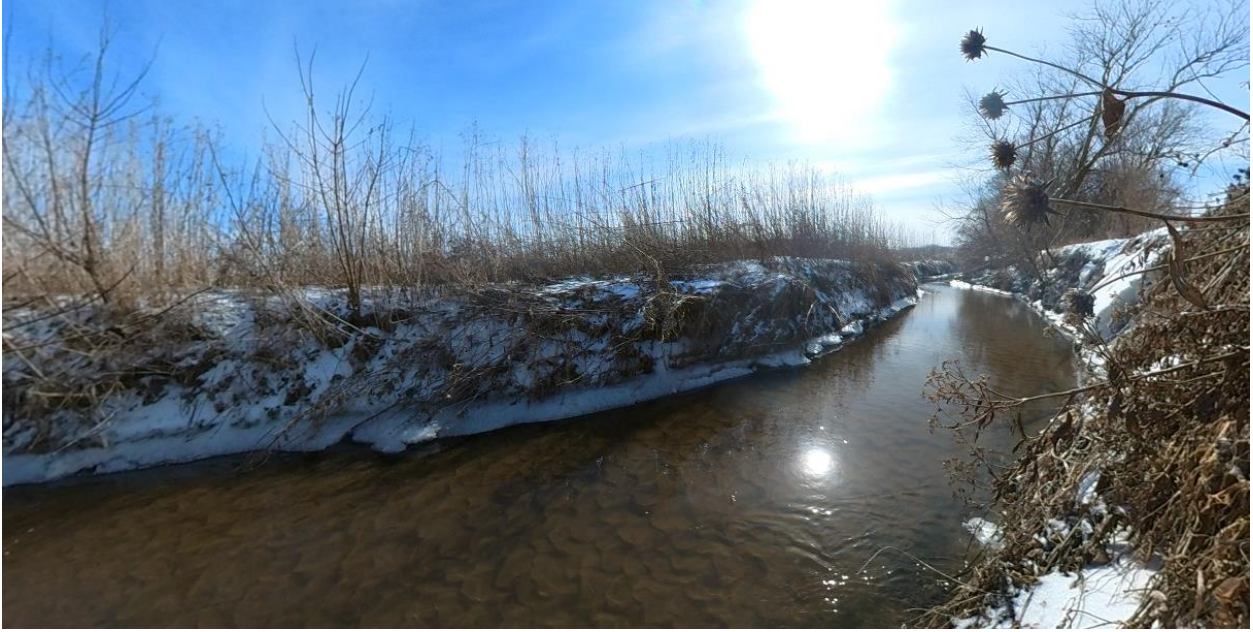
Image 5 - Severe undercut with vegetative overhang
