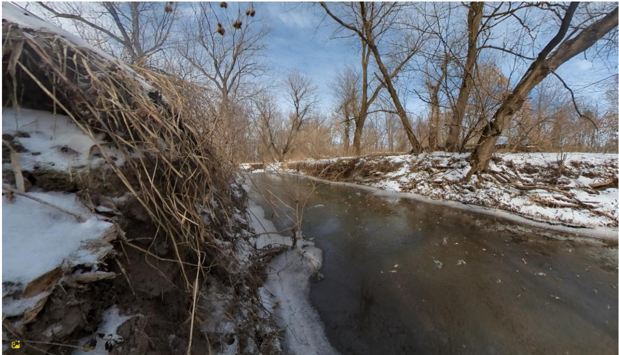
Image 13 - Severe undercut with slump, vegetative overhang, and exposed roots
