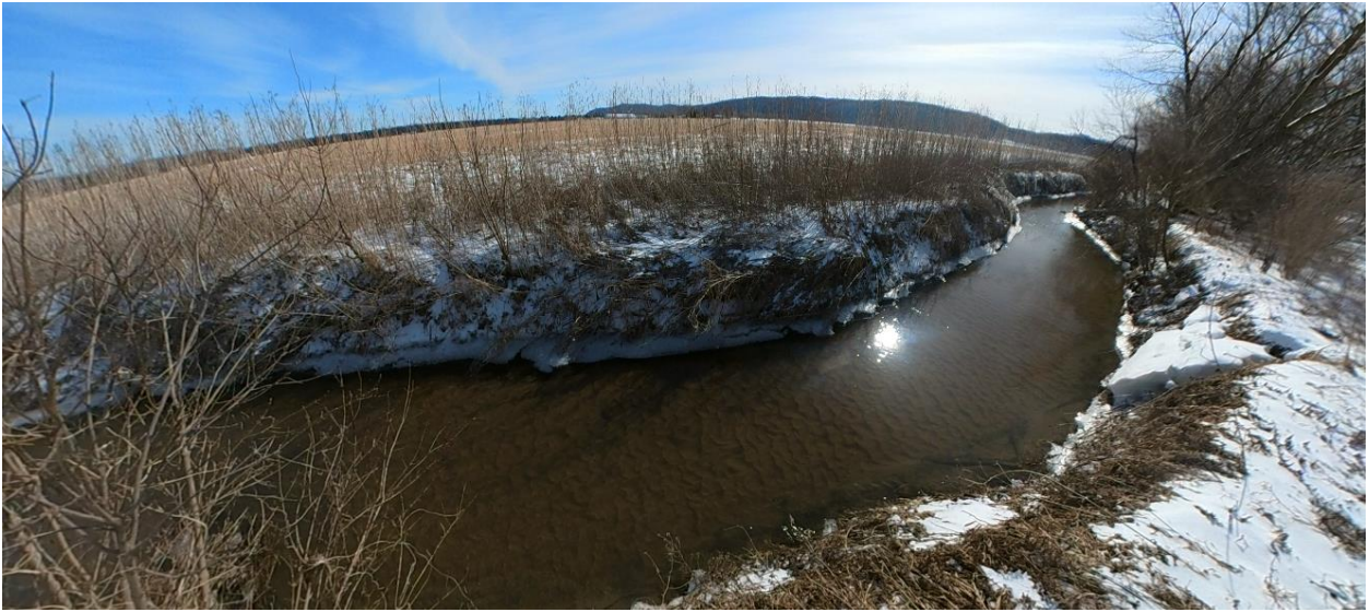
Image 4 - Severe undercut with vegetative overhang
