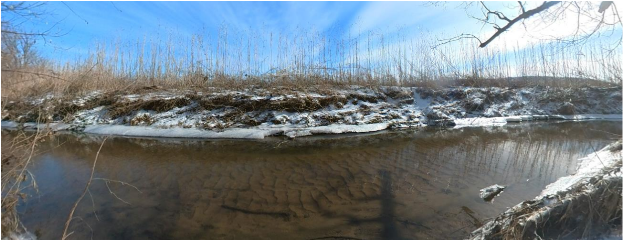
Image 7 - Severe undercut with vegetative overhang
