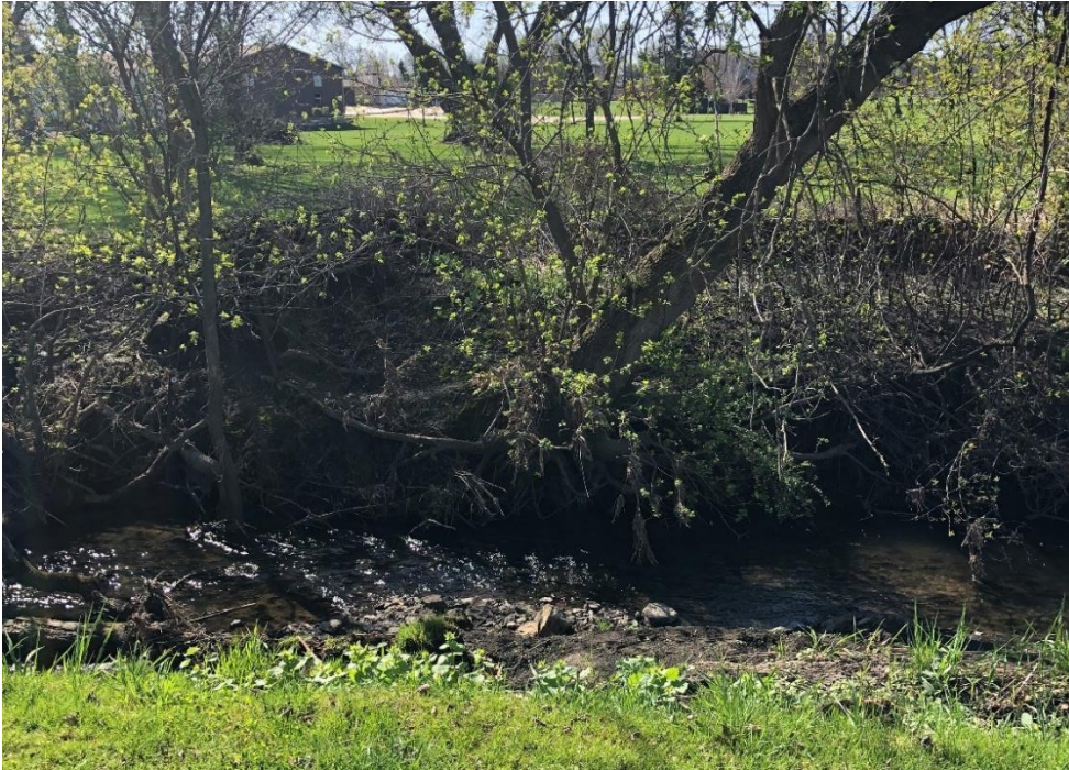
Image 11 – Severe undercut with slump, fallen trees, exposed tree roots, and vegetative overhang.
