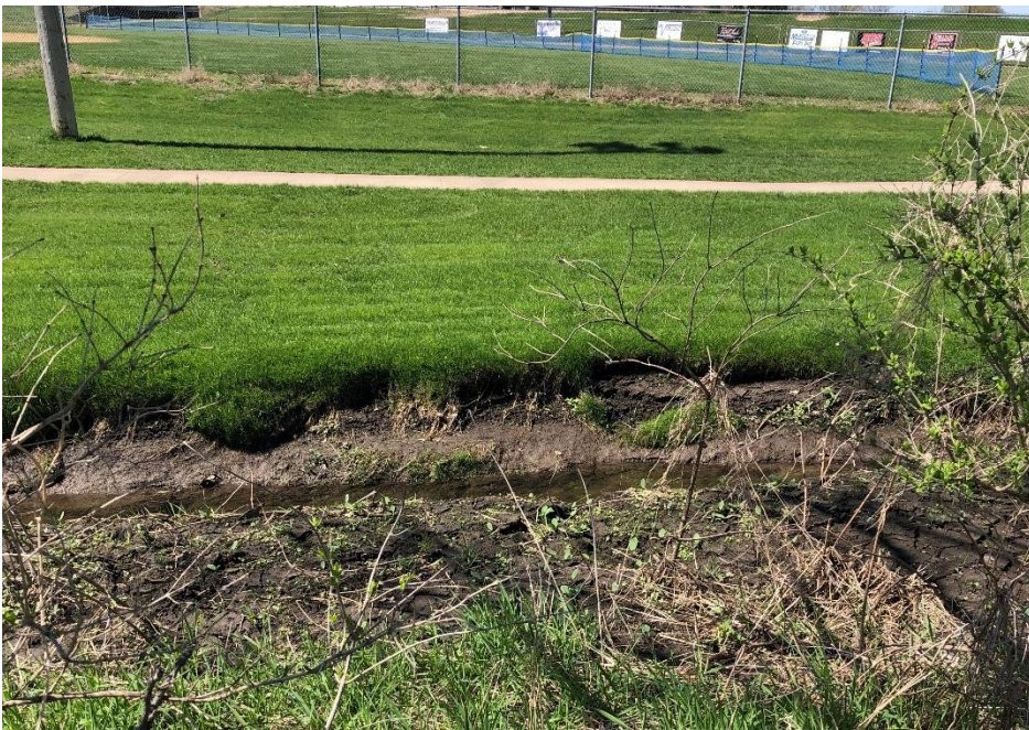
Image 14 – Severe undercut with slump and vegetative overhang.
