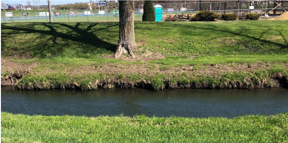
Image 20 – Severe undercut with vegetative overhang.
