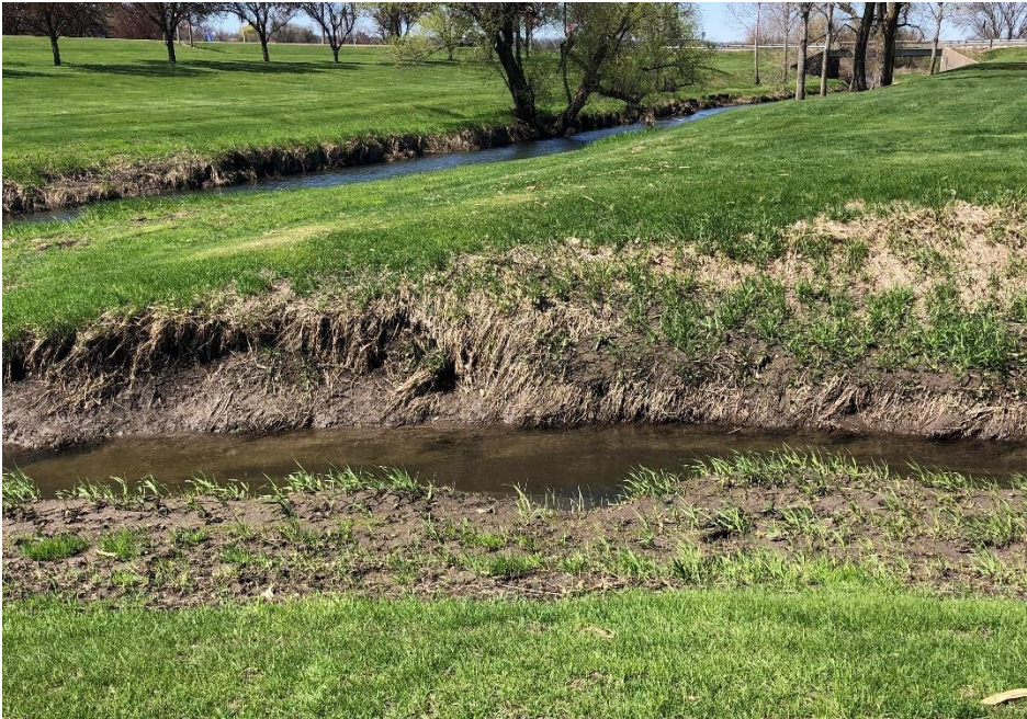
Image 16 – Severe undercut with slump and vegetative overhang.
