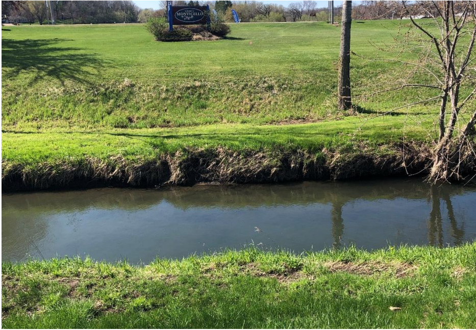
Image 17 – Severe undercut with vegetative overhang.
