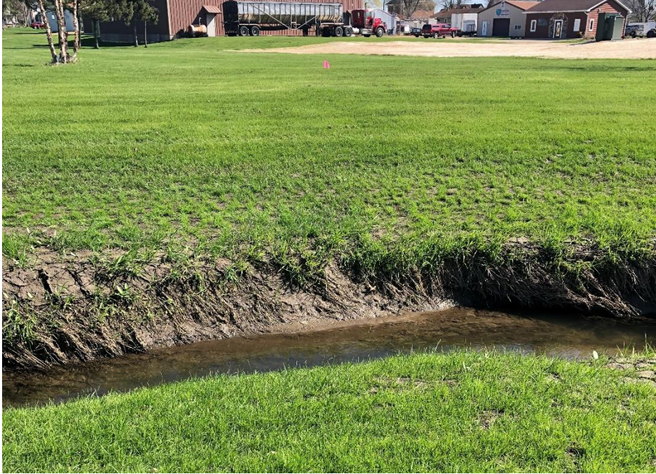
Image 15 – Severe undercut with slump and vegetative overhang.
