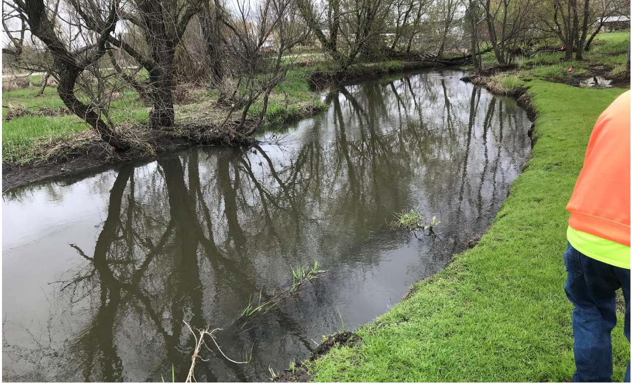
Image 23 – Severe undercut with slump, fallen trees, exposed tree roots, and vegetative overhang.
