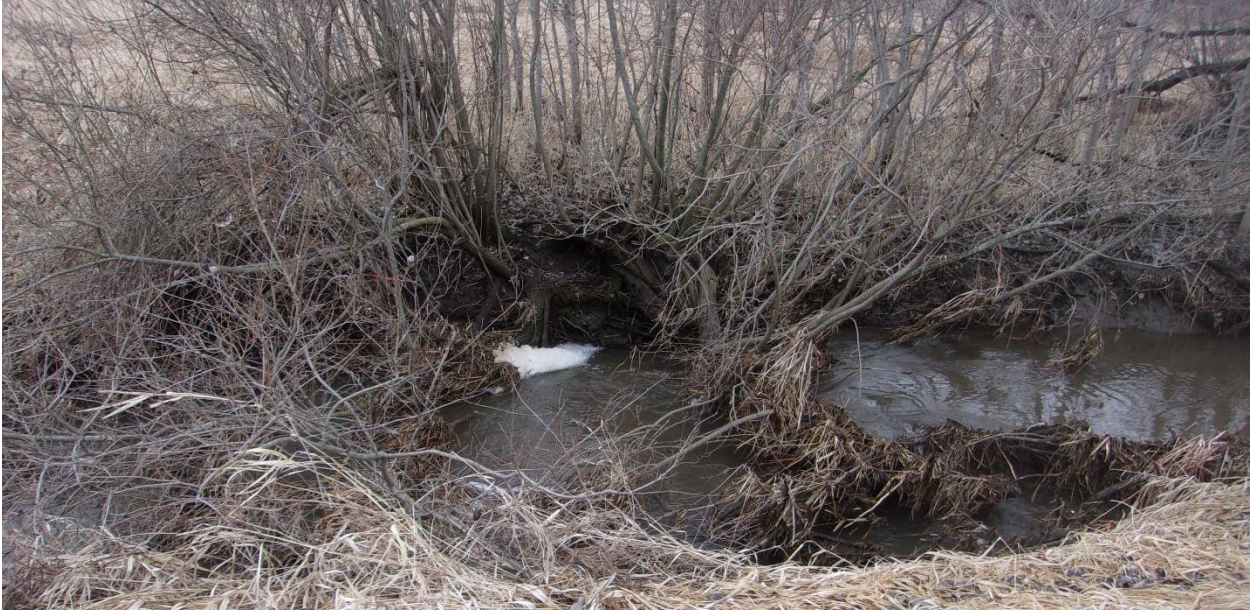
Image 9 – Severe undercut with slump, fallen trees, exposed tree roots, and vegetative overhang.
