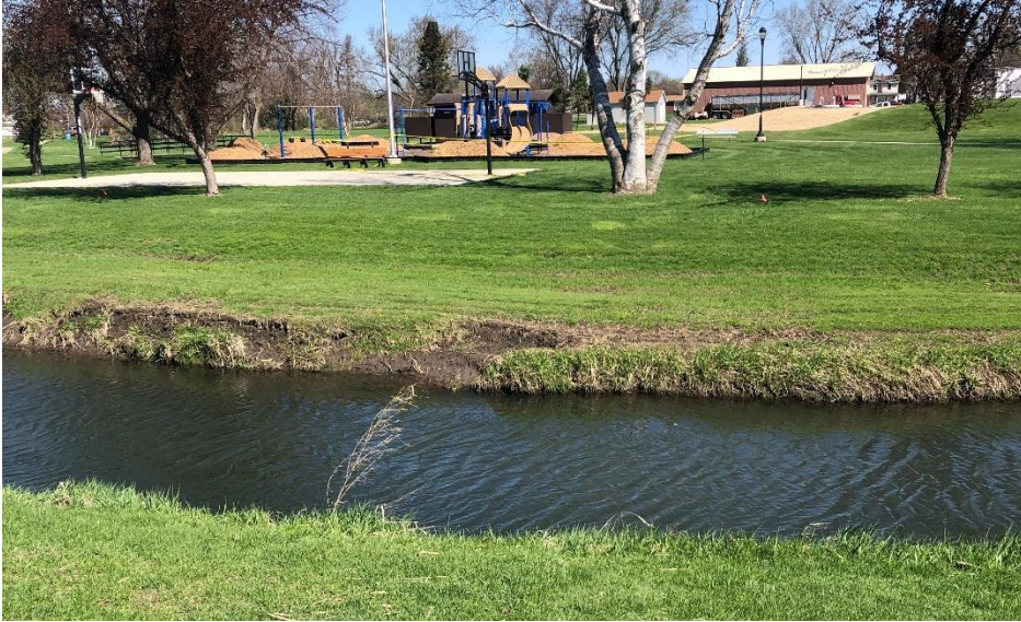
Image 21 – Severe undercut with slump and vegetative overhang.
