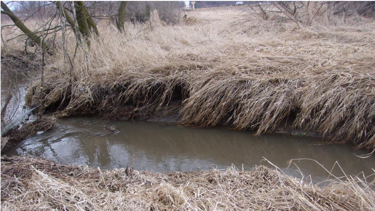
Image 4 – Severe undercut with slump and vegetative overhang.
