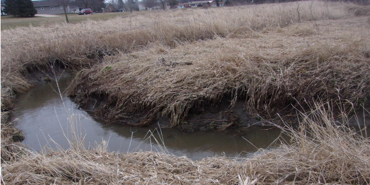
Image 8 – Severe undercut with vegetative overhang.
