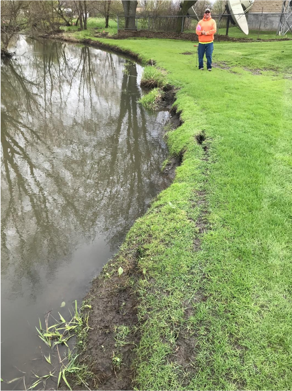
Image 22 – Severe undercut with slump and vegetative overhang.
