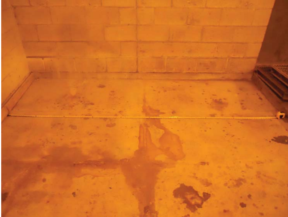
B-1 – NOVISIBLE CRACKS
