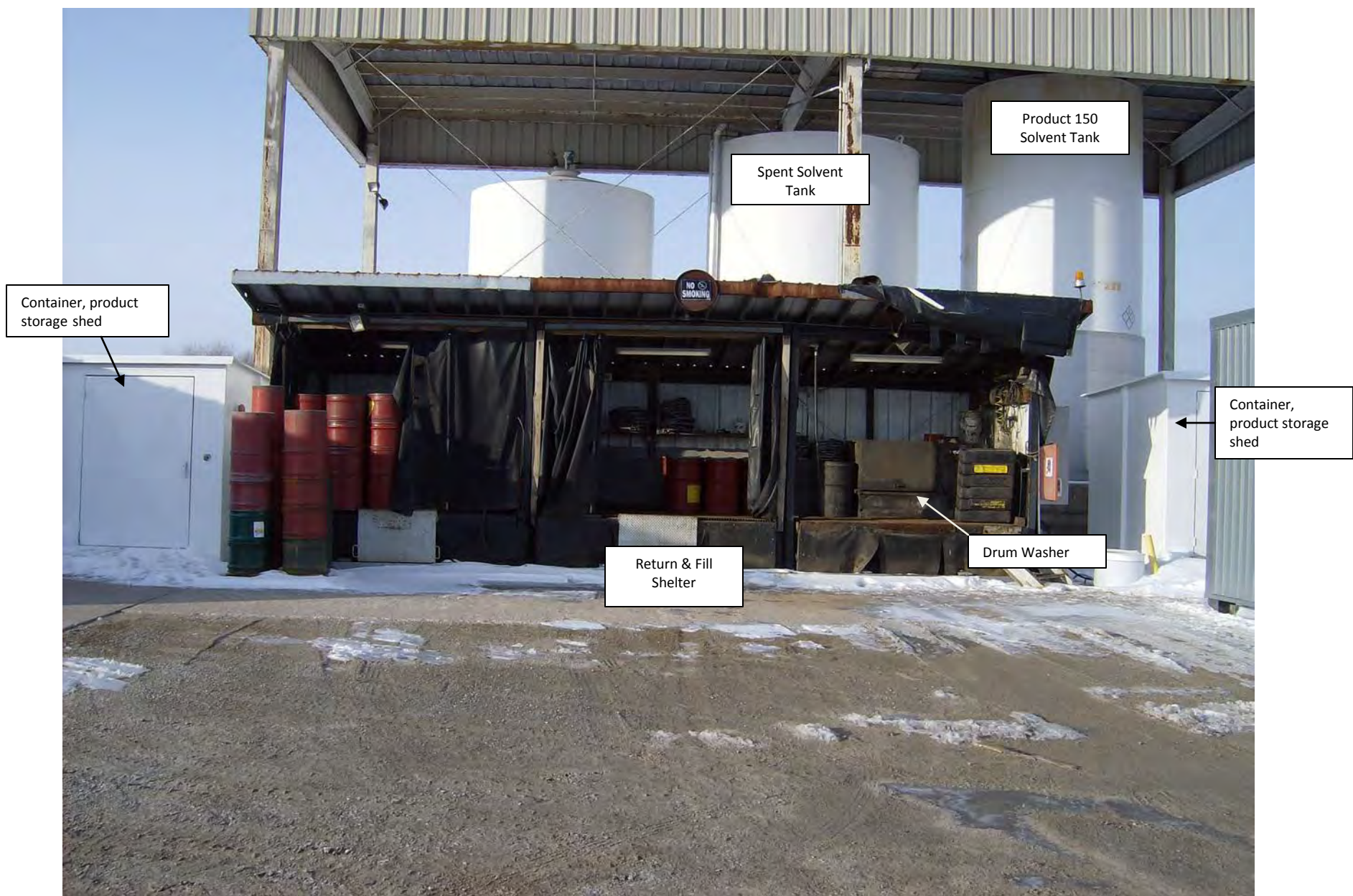
Photo 9. Return and Fill Shelter 2.28.2013
