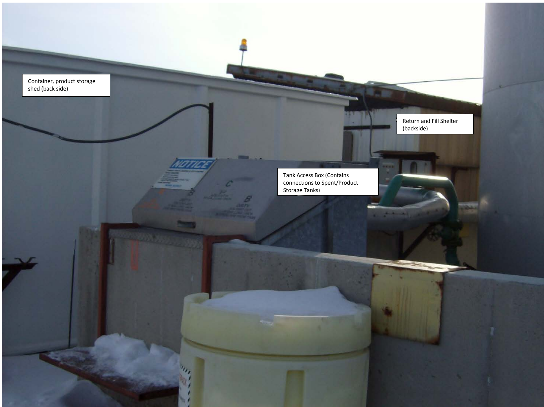
Photo 3. Tank Access Box/Contains Connections to Spent Solvent Tank and Product Tanks by Delivery/Pick-Up Fleet 2.28.2013
