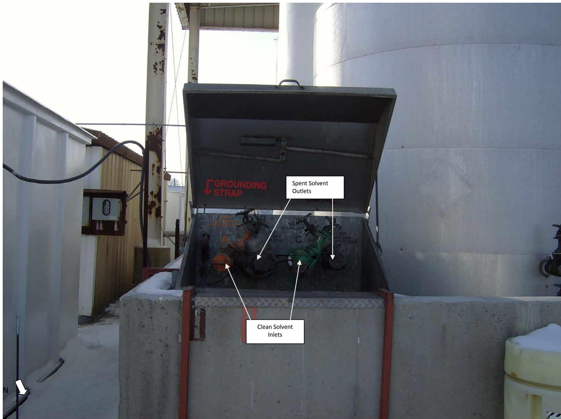
Photo 4. Tank Access Box/Contains Connections to Fill Product Storage Tanks and to Remove Spent Solvent From Tank Used by Delivery/Pick-Up Fleet 2.28.2013
