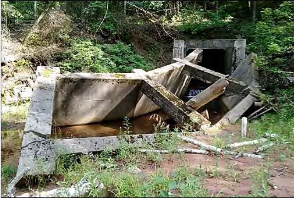
Figure 3. Existing Box Culvert and Collapsed Channel Side Walls, View Southeast
