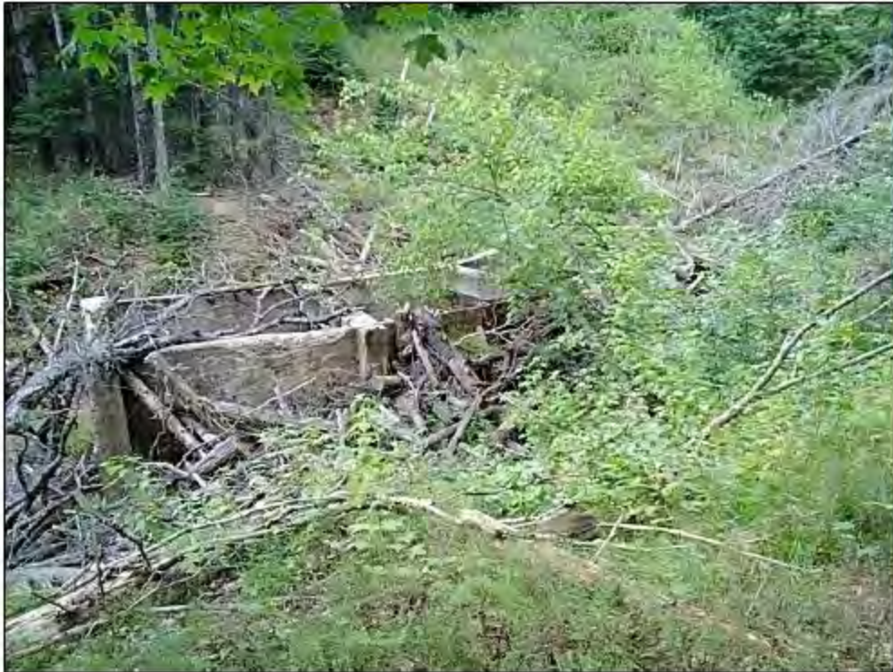
Figure 7. Excessive Slope and Culvert in Little Balsam Creek South of Trail, View Northwest
