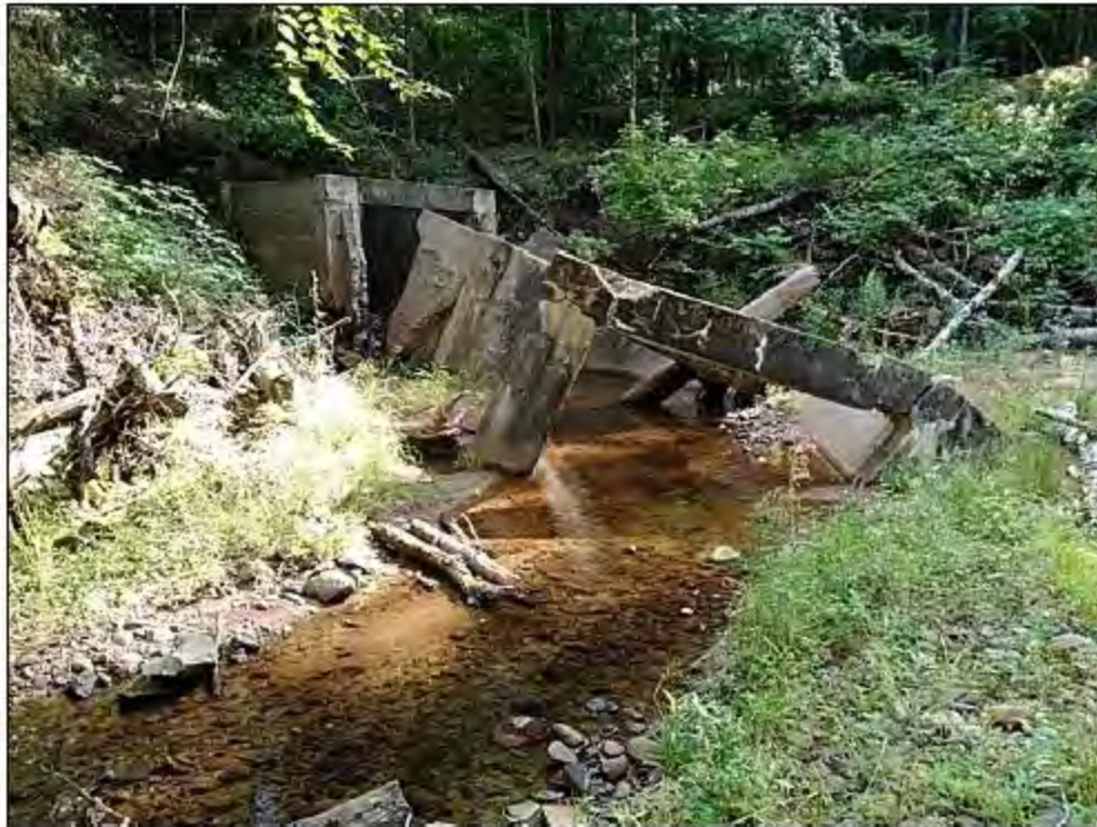
Figure 5. Excessive Slope and Culvert in Little Balsam Creek North of Trail, View Southwest
