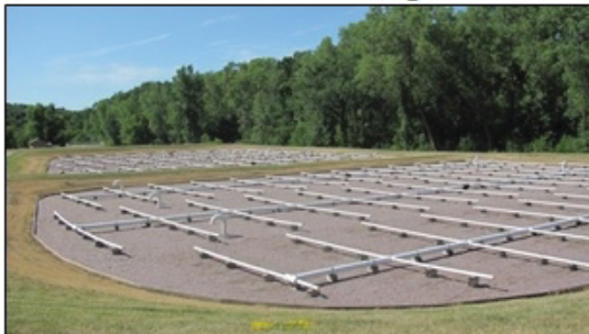
Well-Maintained Recirculating Media Filter
