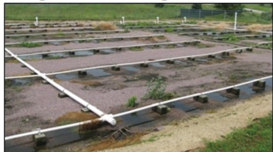
Neglected Recirculating Media Filter
