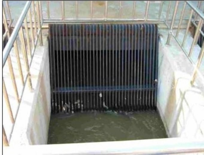
Manually Cleaned Bar Screen
