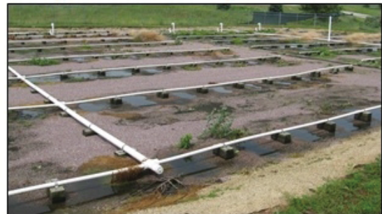
Neglected Recirculating Media Filter
