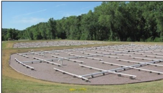
Well-Maintained Recirculating Media Filter
