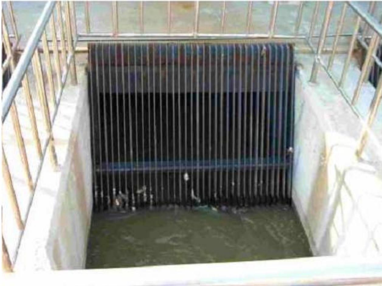
MANUALLY CLEANED BAR SCREEN
