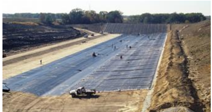
Installation of a compacted clay and geotextile liner at a landfill site in Wisconsin.
