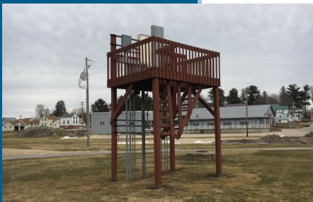
Elevated electrical panel at the Pecatonica River Trails Campground Photo taken by Michelle Staff
