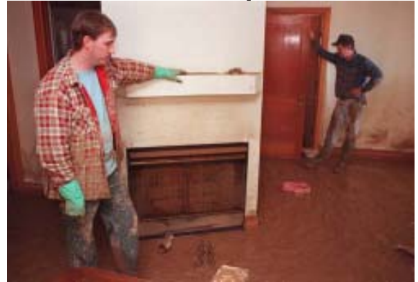
-Surveying the damage
