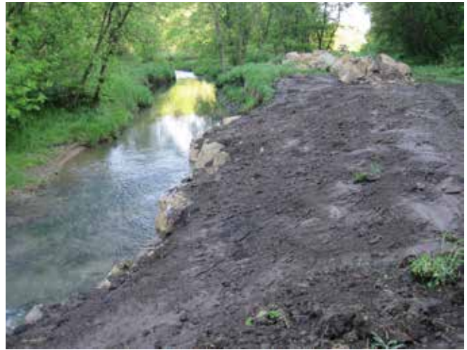
Stabilizing a stream bank using large riprap rock and then sloping the stream bank on the Knapp Creek project located in Crawford County.
