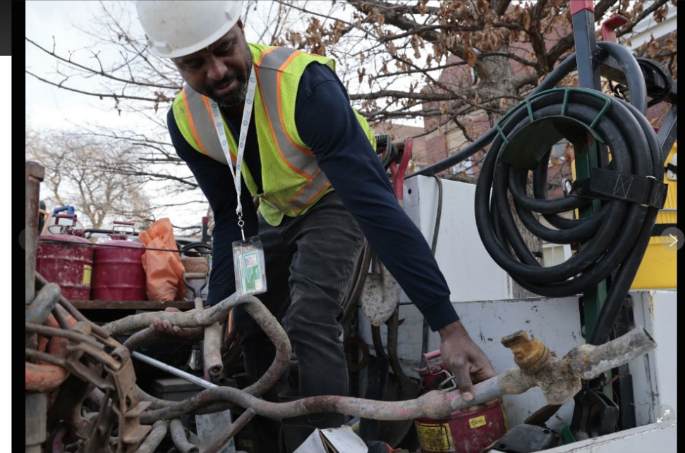
1 of 3 | Blackhawk Sewer & Water contractor Khalid Waarith holds a lead pipe that was extracted in Chicago on April 10, 2023. Lead pipes that carry drinking water are a major source of exposure to the metal and the damage is usually permanent. (Antonio Perez/Chicago Tribune via AP)
