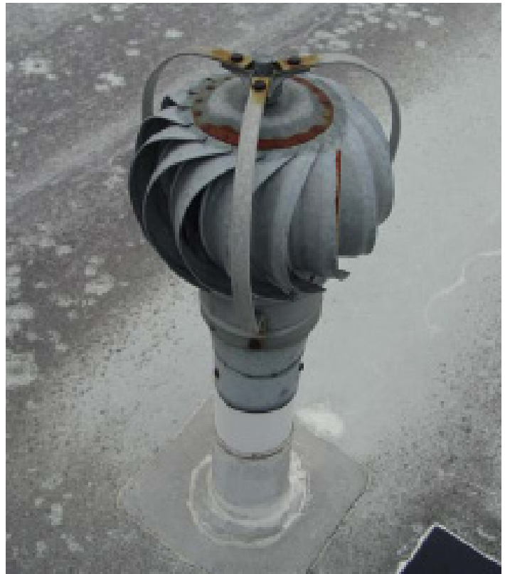
Figure 16. Roof vents fitted with wind turbines provide slight depressurization of the sub-slab area and prevent the buildup of contaminants beneath the building.
