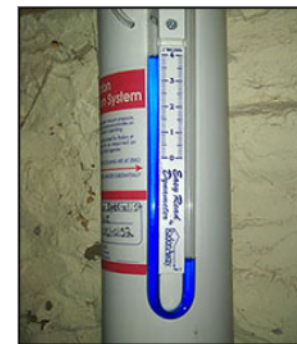
The manometer measures suction created by the vapor mitigation system fan. The uneven levels of the liquid indicate the system fan is running but cannot be used exclusively to determine the effectiveness of the system.
