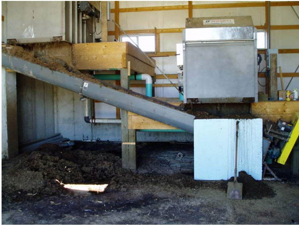
Figure 4.1 Integrity Co., Solids Separators
