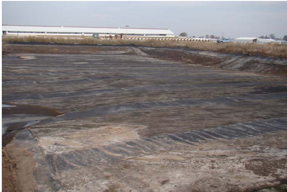
Figure 3.1 Permeable Cover on Lagoon #2, Kewaunee County Farm
