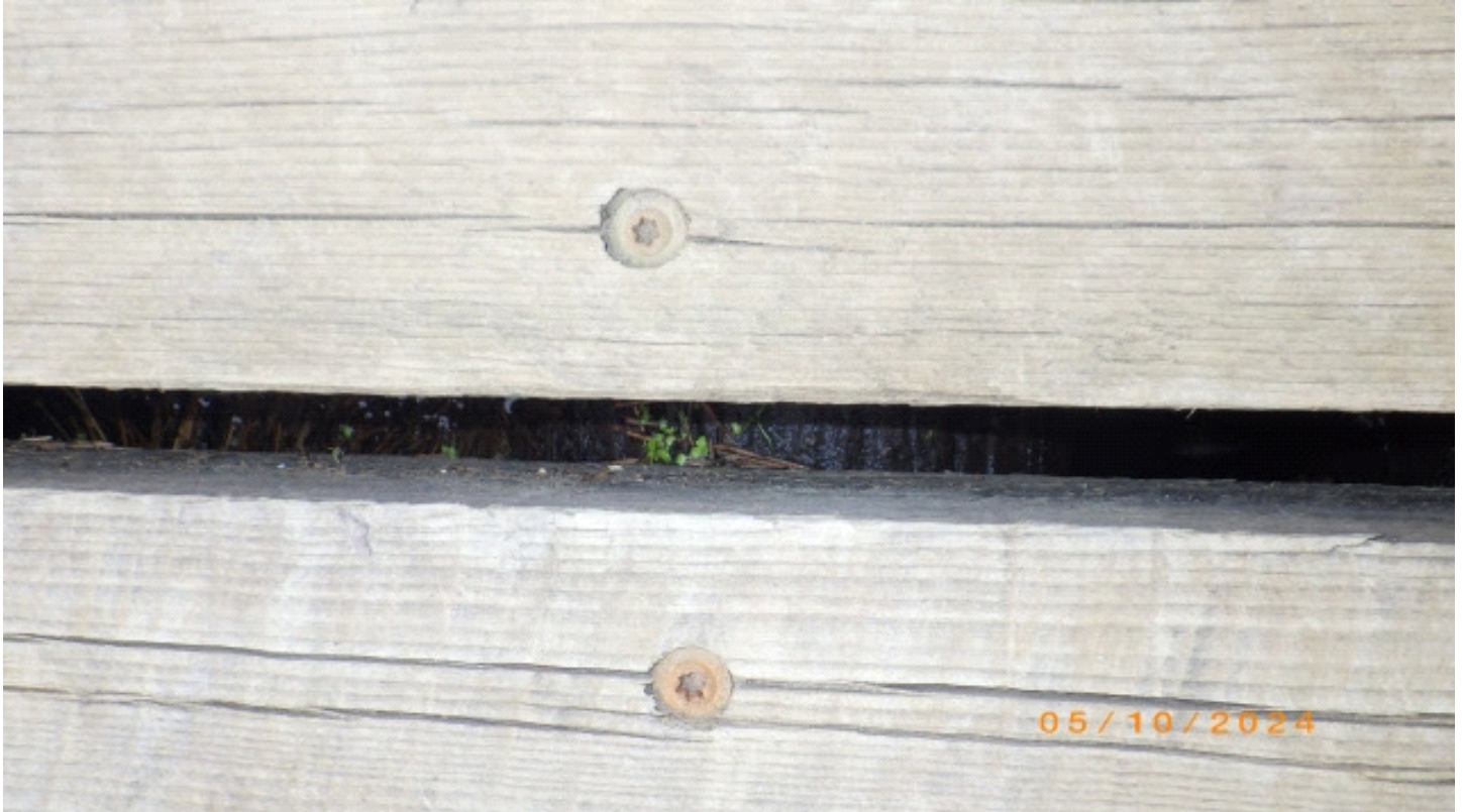
Very decayed timber superstructure.
