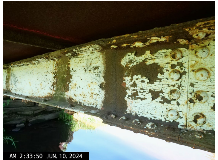
Girder Offset Welded Spice next to Riveted Spice
