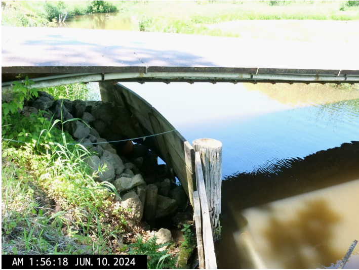
South Abut., Retaining Wall Timber Pile Deterioration
