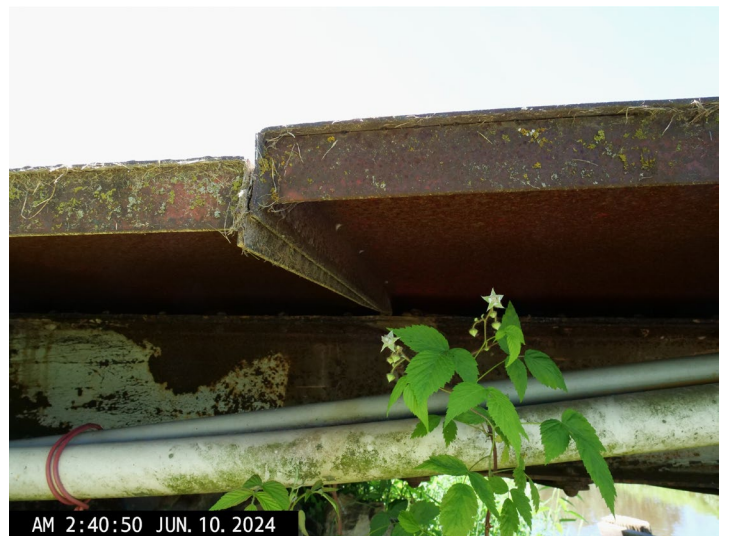
Bent Down Deck Panel
