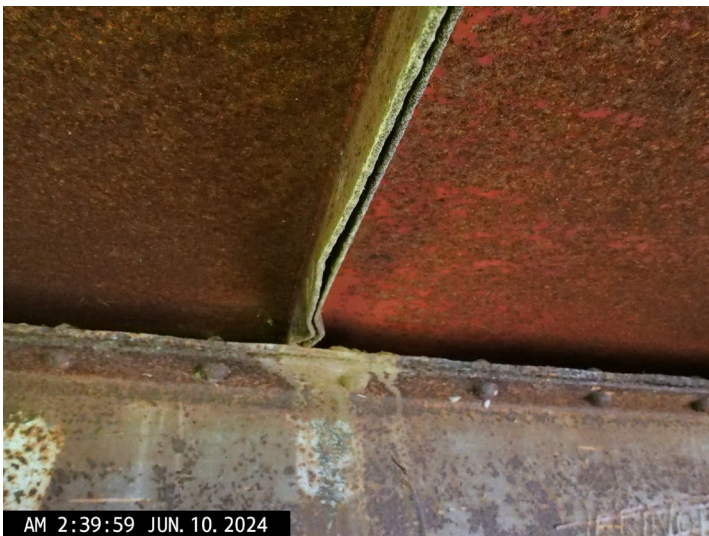
Failing Angle Iron Deck Panel Support
