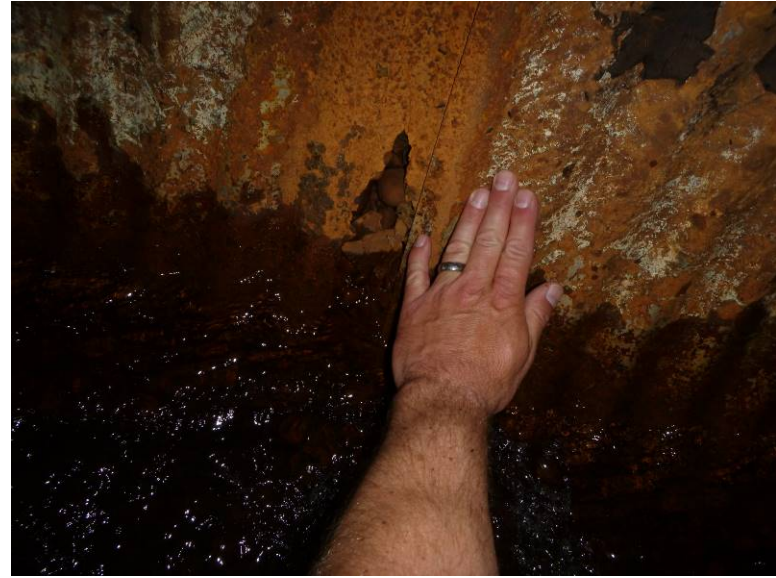
Same rust damage.
