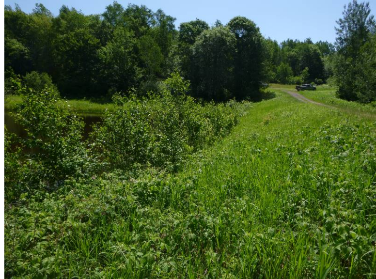
Woody growth on US embankment requires removal.
