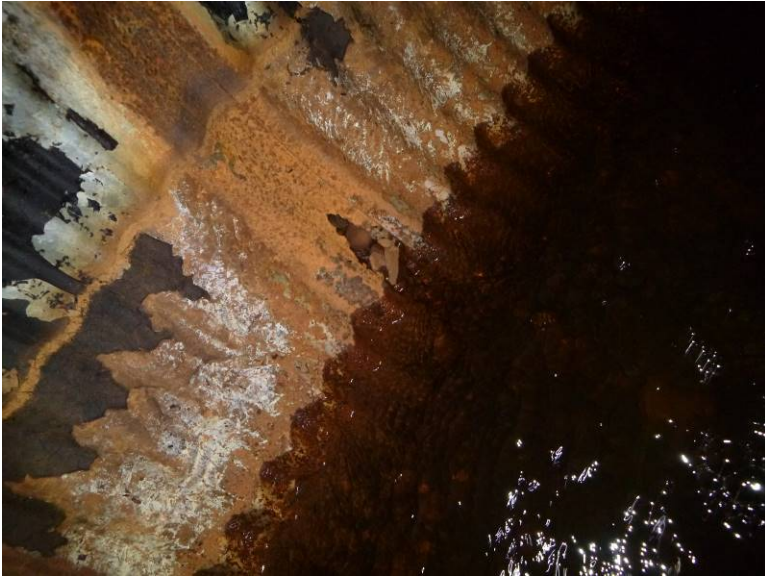
Rust damaged pipe. Approx. 20' in from outlet.
