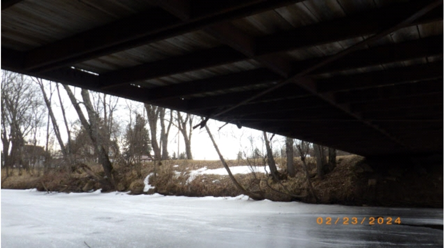
Damage cross bracing with debris in deck.
