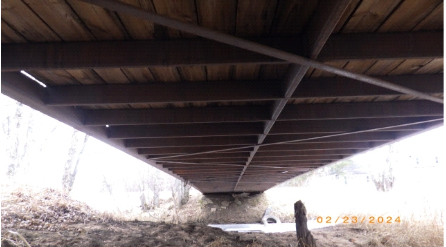
Bottom of deck, with debris in deck.
