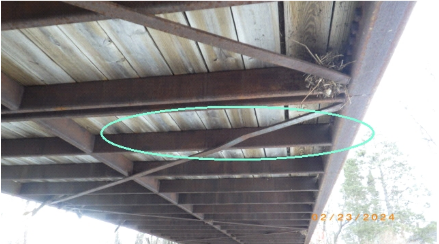
Damage cross bracing with debris in deck.
