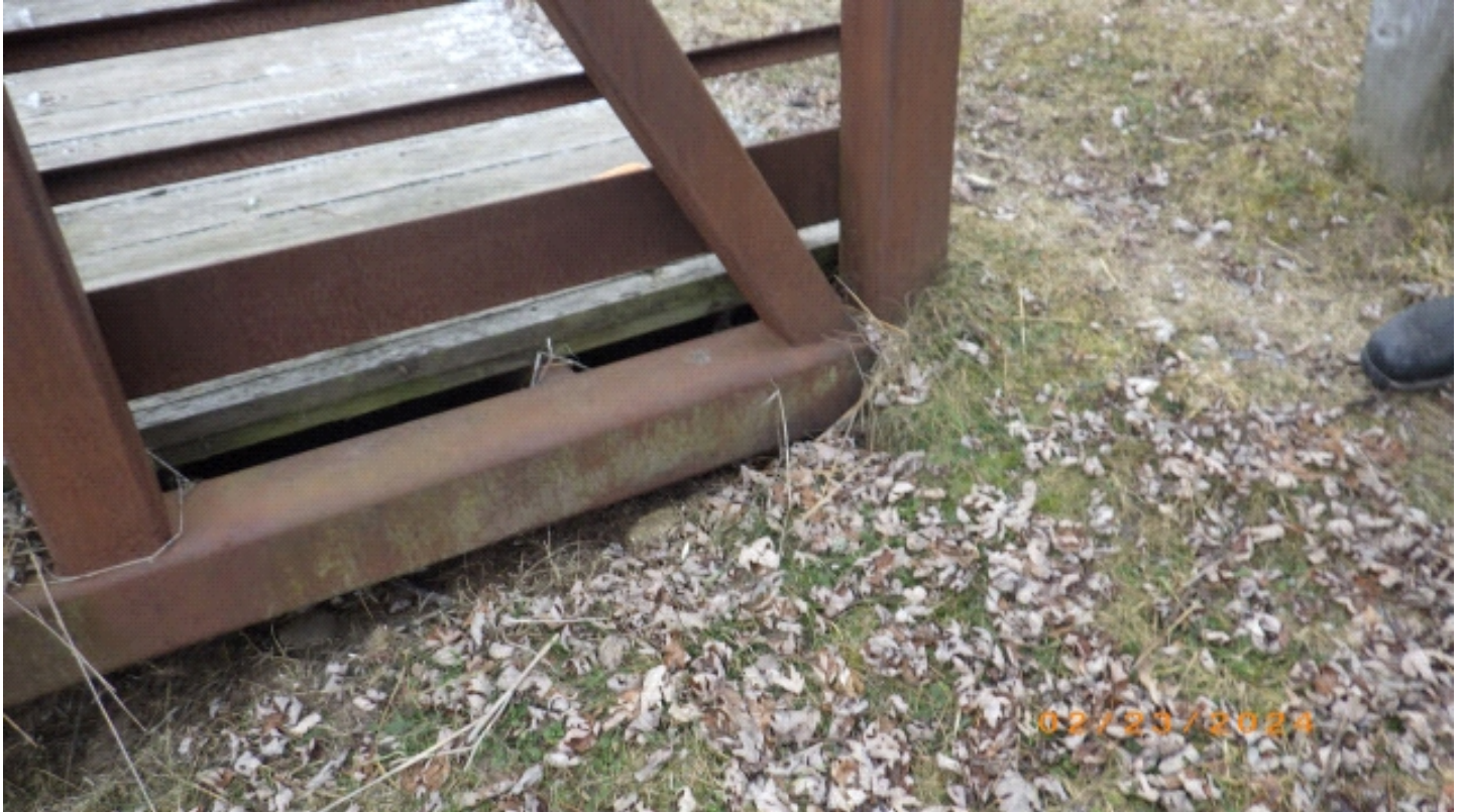
NW bearing, clean as it is buried, which is bad.
