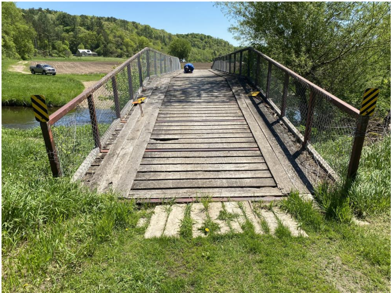
Approach from the north. Groomers are unable to cross this bridge and take a river crossing instead.
