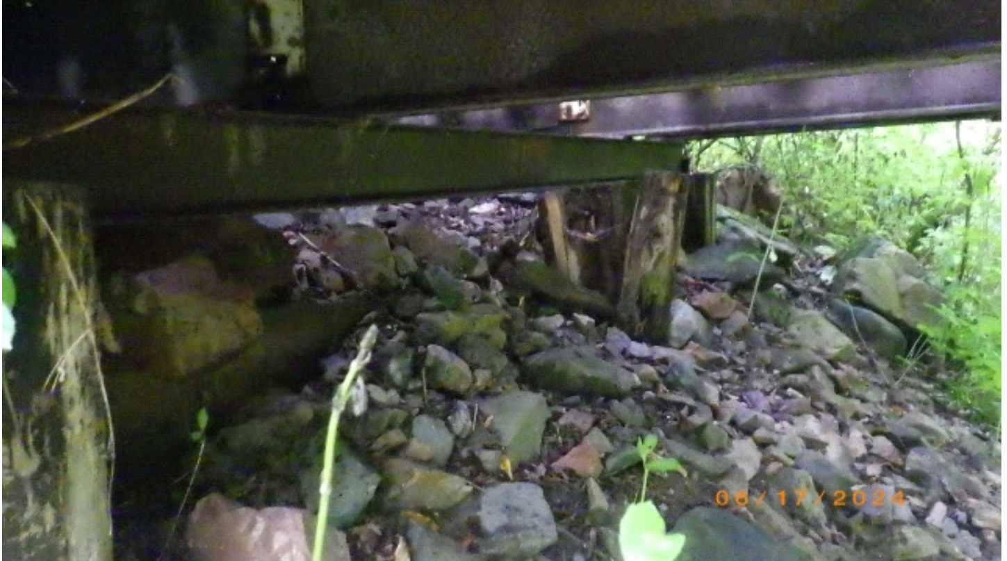
Failed East Pier
