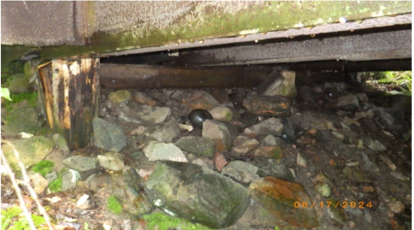
Failed West Pier
