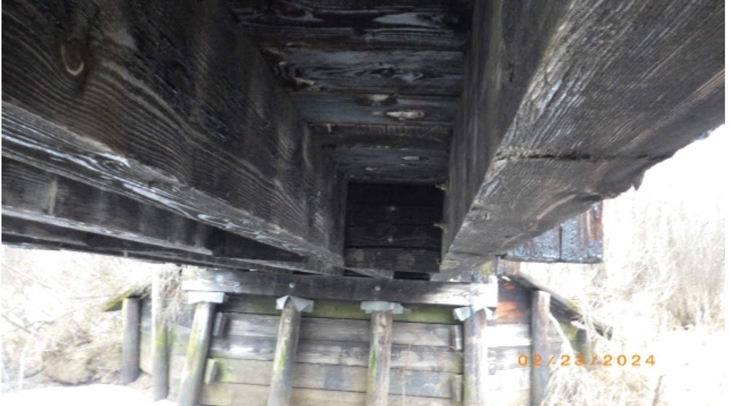
Sag in pile cap.
