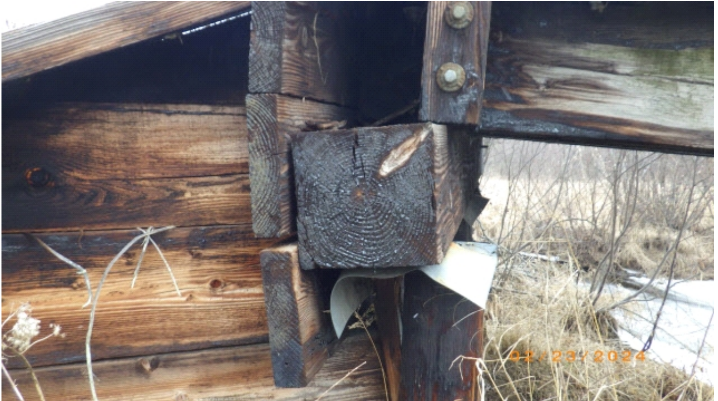
Pile cap pushed off the piles.
