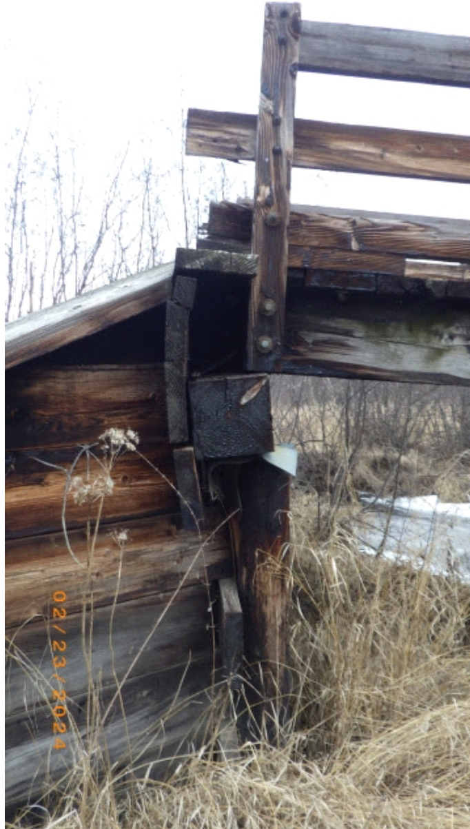
Pile moving independent of piles caps.
