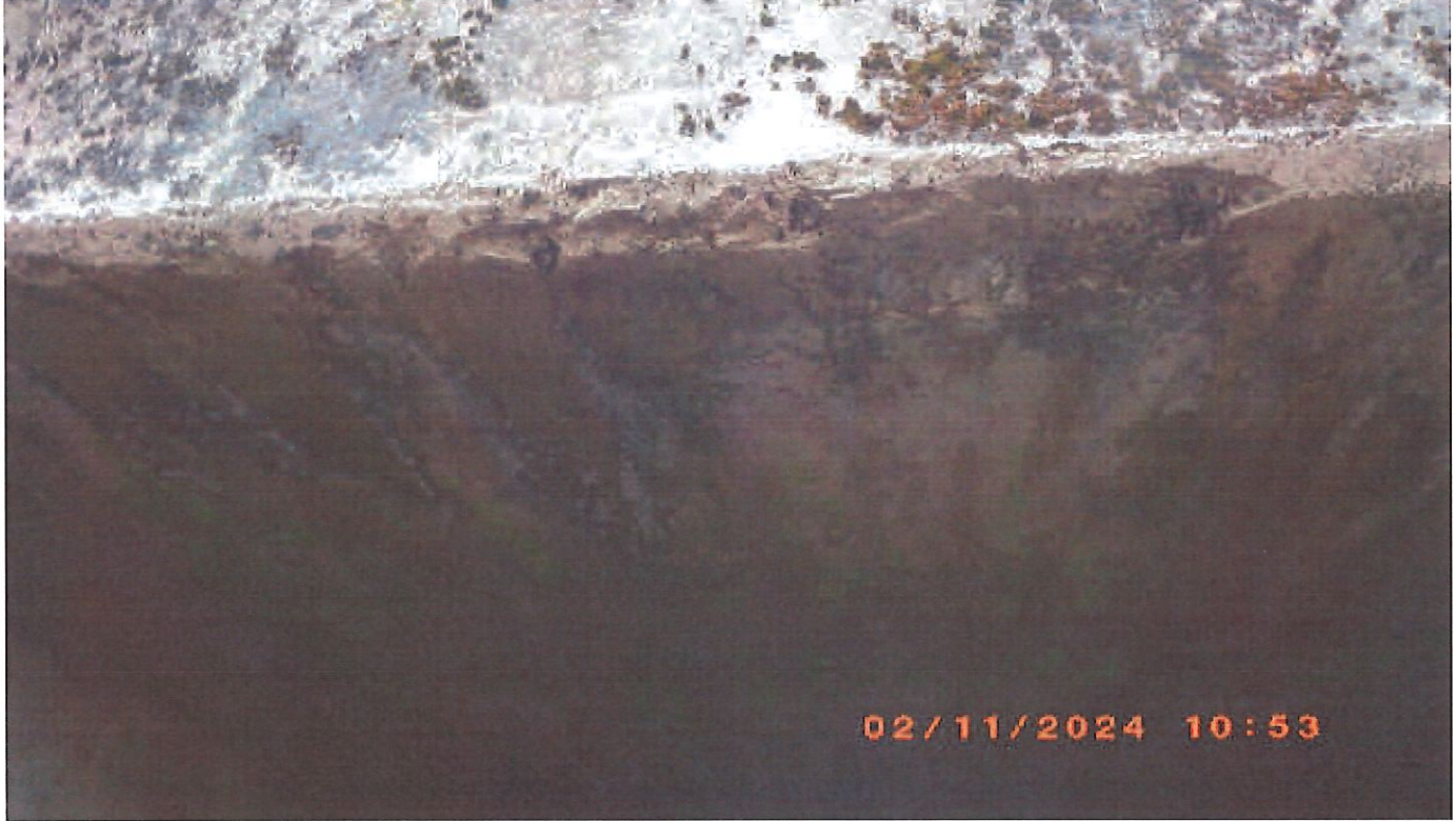
Spall on top of box, east end
