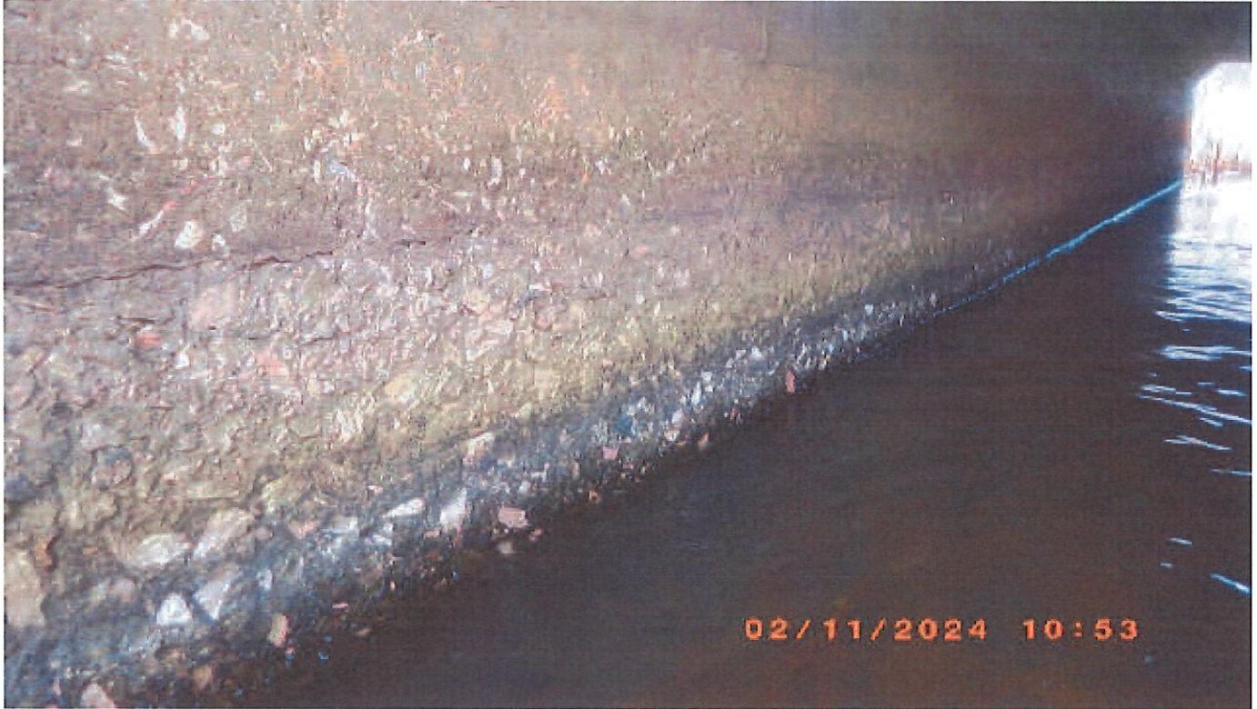
CS2 scaling on wetted perimeter of box
