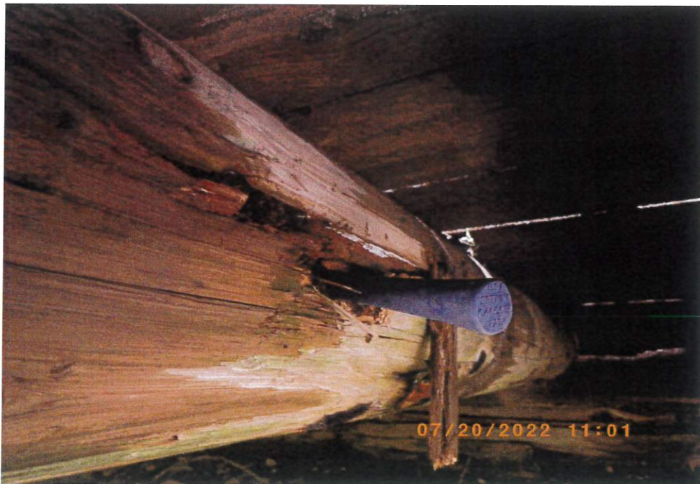
3rd girder from upstream completely rotten at 1/4 point.
