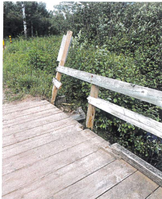
NE rail section destroyed from groomer impact
