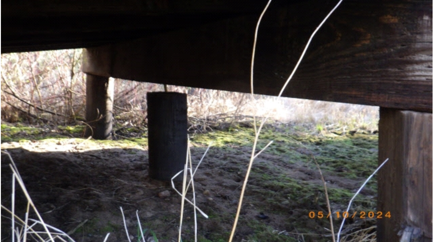
P1 and P2 gap at middle pile, fill space to protect pile cap under load.
