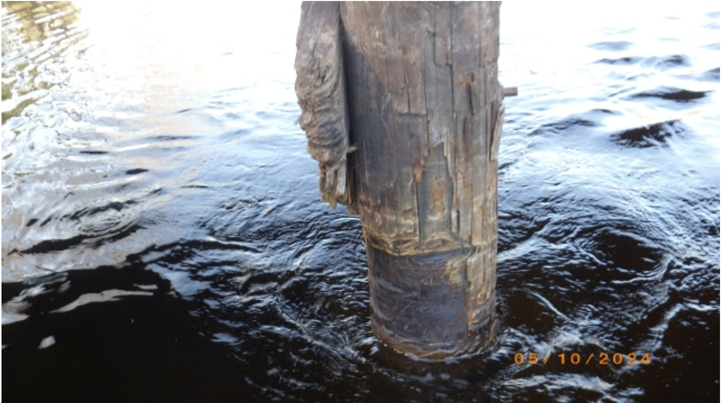
Wear from Ice and Debris on upstream pile in channel, typical.
