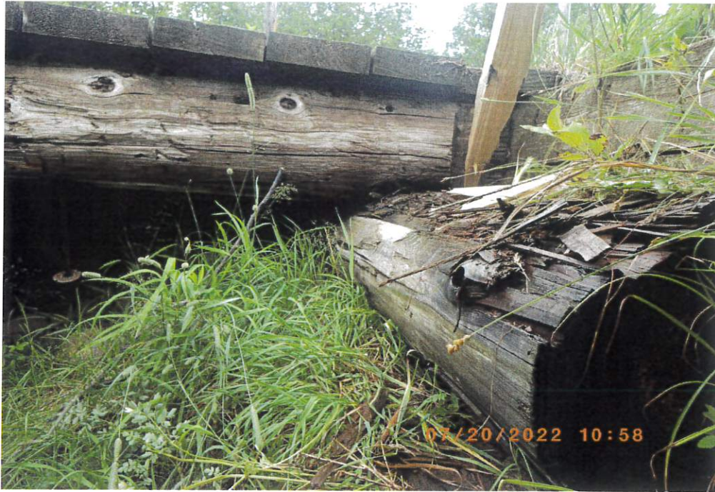
East end of north sill, rotten and delaminated
