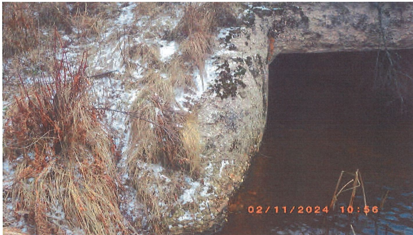
NW wingwall section loss
