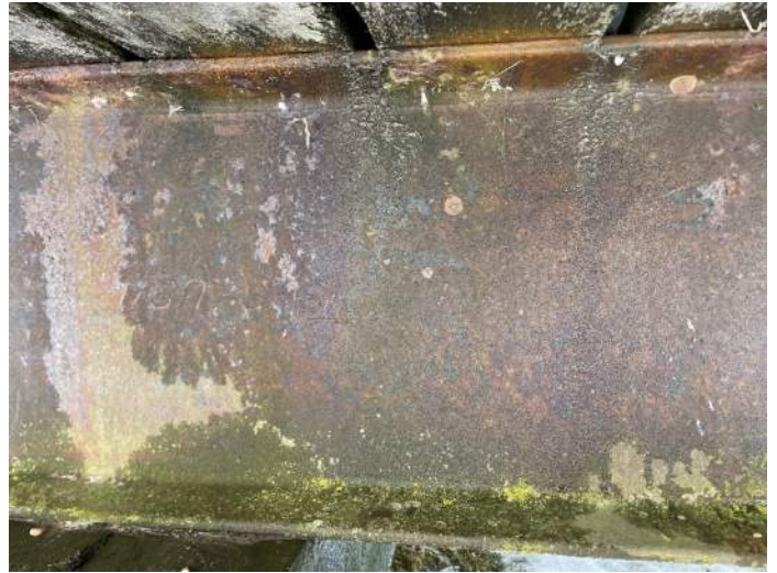
Timber and girder condition at contact.
